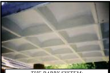
THE PARRY SYSTEM: Coffer underside of upper floor installed without need of timber shuttering and reducing the quantity of concrete by half
