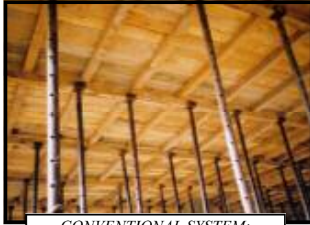
CONVENTIONAL SYSTEM: The large area of shuttering used to support a floor of reinforced concrete while it sets consumes copious amounts of timber
